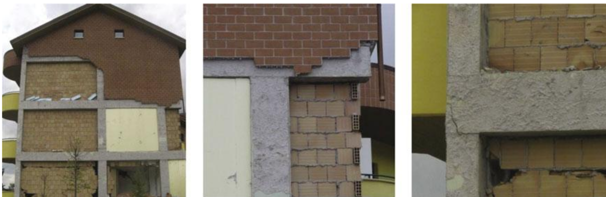
Fig. 8. Out-of-plane failure of the outer leaf due to the lack of anchoring systems to the inner leaf and insufficient width support over the beam, the 2009 L'Aquila earthquake (Vicente et al. , 2012)
