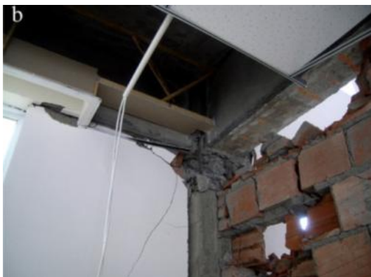
Fig. 19. Failure of wall corner and shear failure of column; the 2008 Wenchuan earthquake (Zhao et al., 2009)
