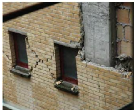
Fig. 5. Diagonal cracking in piers, the 2009 L'Aquila earthquake (Ceci et al. , 2010)
