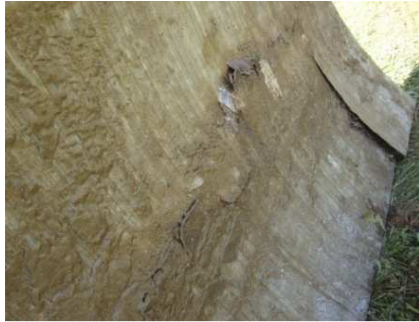
Fig. 2. Longitudinal crack in pipes
