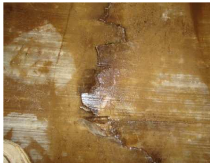
Fig. 3. Longitudinal crack in pipes
