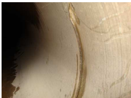
Fig. 4. Circumferential crack in pipes
