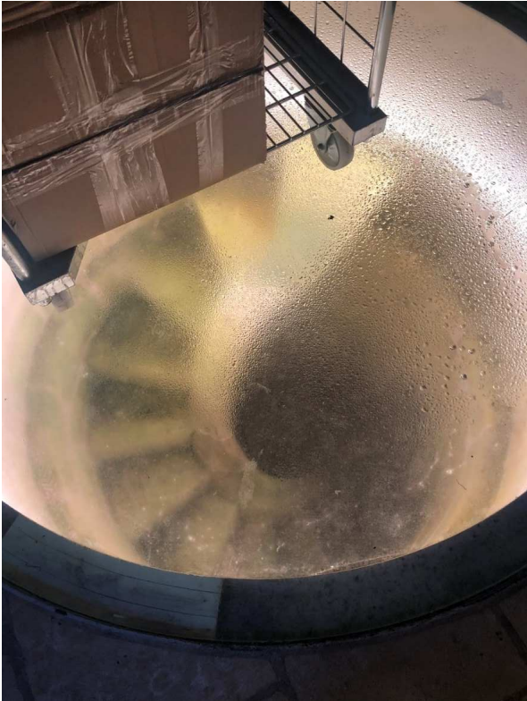
Fig. 18. Glass panel placed in the floor to provide a view of an original staircase uncovered during the restoration works.
