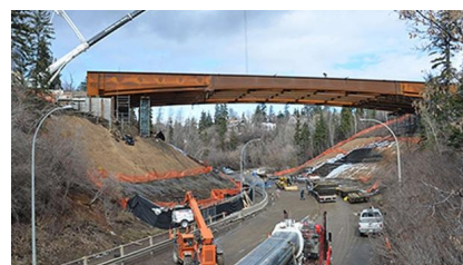
Fig. 6. Aerial view of the beams under a failed position ( https://edmonton.ctvnews.ca/damaged-girders-on-102-ave-bridge-repaired-to-be-reinstalled-1.2375088 ).
