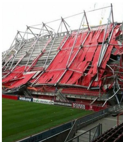
Fig. 3. Local view of the collapsed roof ( http://www.bbc.com/news/world-europe-14063640 ).
