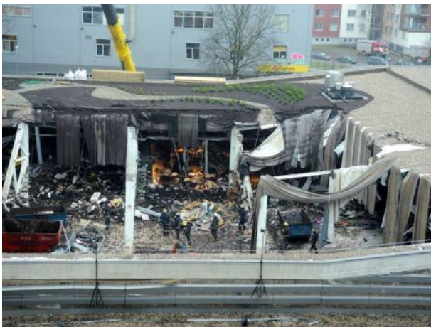
Fig. 4. Global view of the Maxima collapsed roof ( http://dailymail.co.uk/news/article-2511652-Latvia-supermarket-roof-collapse-kills-37-Riga.html ).
