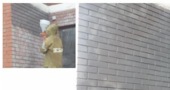
Fig. 3. Application of the silicate top coat with a spray gun and general view of the walls after painting
